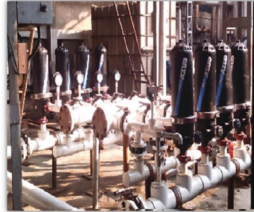
JAIN TEXTILE INDUSTRIES LTD, GURGAON HARYANA MODEL : 2" X 8 FLOW RATE : 50 m 3 /h FILTRATION GRADE : 20 MICRON APPLICATION : BOILER WATER
