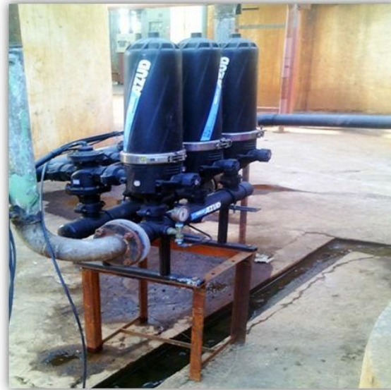
LANCO POWER LIMITED MAHARASTRA MODEL : 203/3 FX DLP FLOW RATE : 42 m 3 /h FILTRATION GRADE : 50 MICRON APPLICATION : PROCESS WATER
