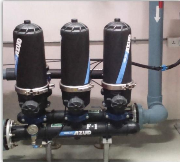
MYLAN PHARMA (UNIT 8) VISAKHAPATNAM, AP MODEL : 203/3FX FLOW RATE : 40 m 3 /h FILTRATION GRADE : 50 MICRON APPLICATION : PRE-FILTRATION
