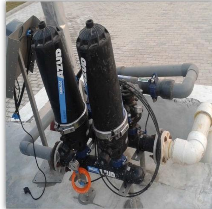
MUNJAL FARM HOUSE NEW DELHI MODEL : 202/3 FX FLOW RATE : 40 m 3 /h FILTRATION GRADE : 100 MICRON APPLICATION : PROCESS WATER PRE FILTRATION
