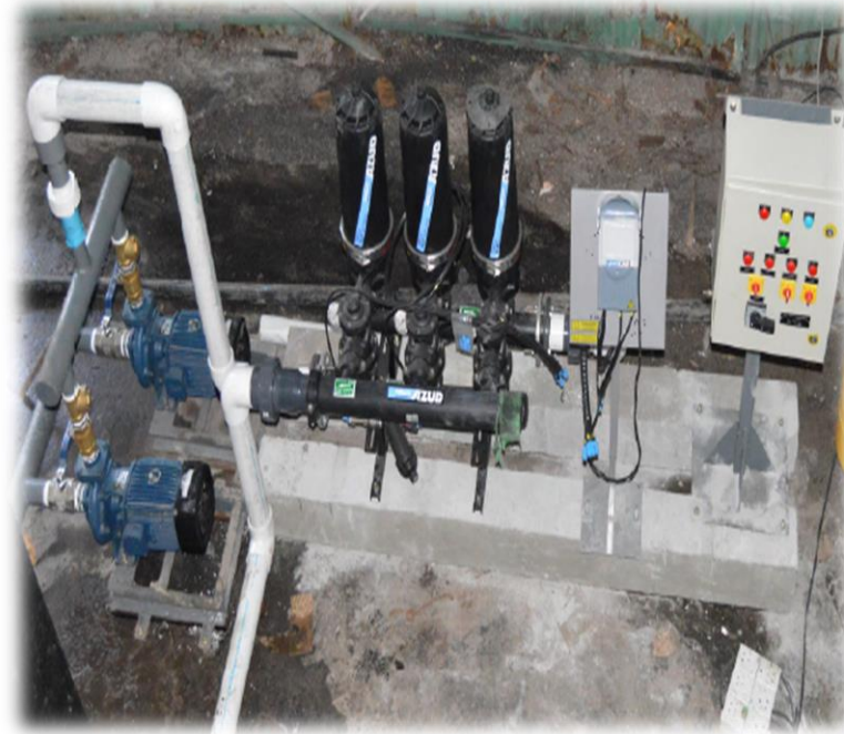
EROS GROUP NEW DELHI MODEL : 201 FLOW RATE : 14 m 3 /h FILTRATION GRADE : 50 MICRON APPLICATION : PRE FILTRATION
