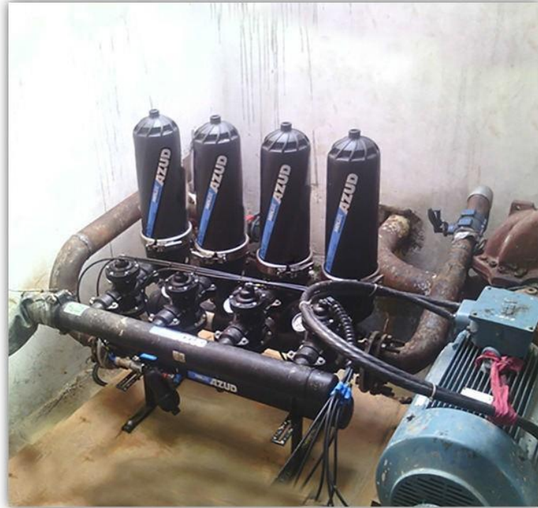
RIMJHIM STEEL LIMITED, UNNAV, UTTAR PRADESH MODEL : 204/4 FX DLP FLOW RATE : 56 m 3 /h FILTRATION GRADE : 50 MICRON APPLICATION : WATER FILTRATION
