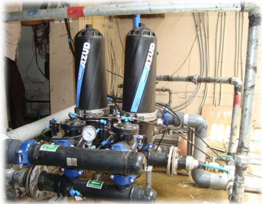
DM HOTEL JORHAT, ASSAM MODEL : 202/3 FX FLOW RATE : 30 m 3 /h FILTRATION GRADE : 20 MICRON APPLICATION : WTP
