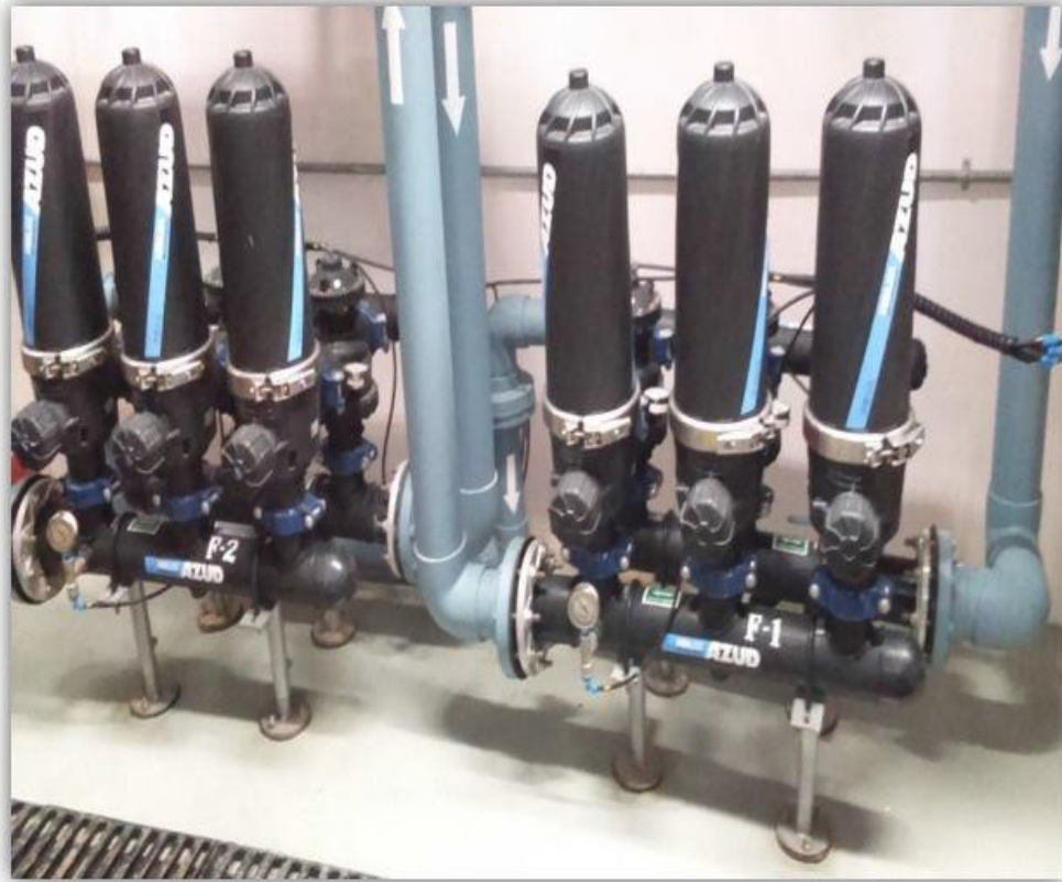
CANADIAN HIGH COMMISSION, NEW DELHI MODEL : 303/4 FX TWO UNITS FLOW RATE : 110 m 3 /h FILTRATION GRADE : 100 MICRON APPLICATION : RAW WATER FILTRATION
